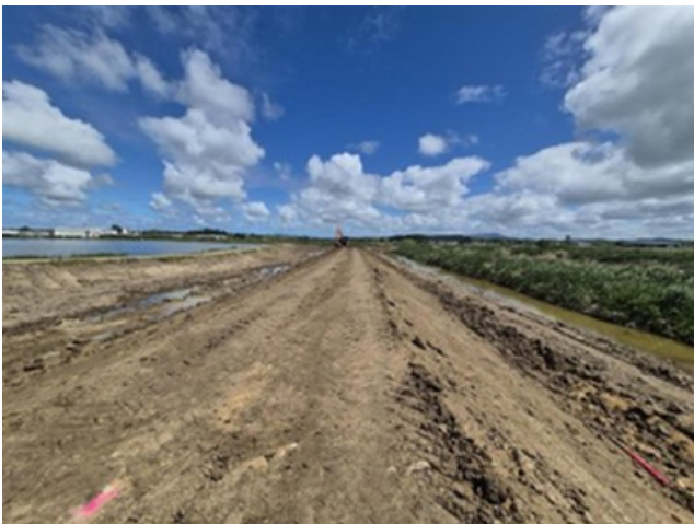
Dargaville wastewater treatment plant flood protection
